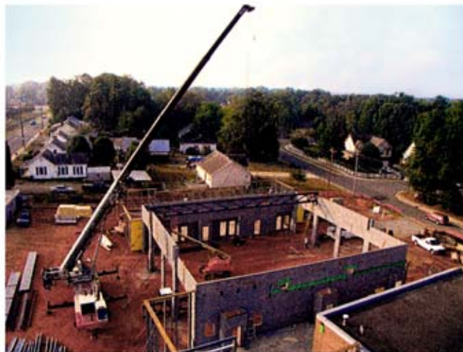
Throughout construction of the new building, Streamline had to maintain all of the station's existing services so it could continue operations. Picture courtesy of the town of Cornelius.
